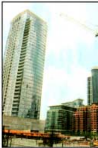
A crane hovers over the construction site at One Museum Park, a 62-story condo to be built at the south end of Grant Park.
